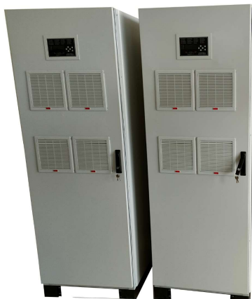
Three phase output 2*100 kVA
